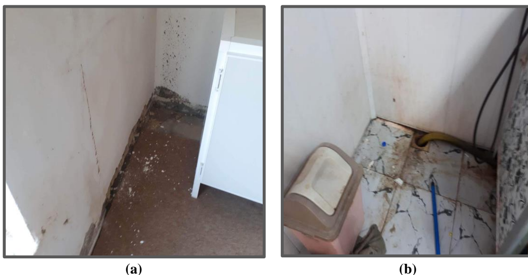
Figure -1 (a) and (b). Show the damp indoor building signs which are contaminated by a moldy odor in some places. with a dark spot in the ceiling, wallpaper, archives and bathrooms.
